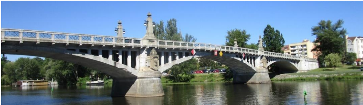
Fig. 2: View of the historical bridge at Nymburg (Czech rep.) with art-neveau artistic features
